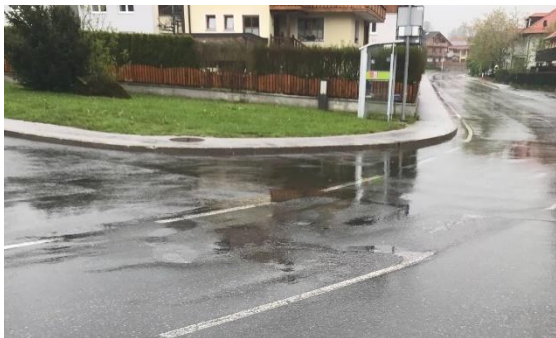
Figure 37: Standing water at the edge of the road and on uneven surfaces (Source: Salzburg Research)
