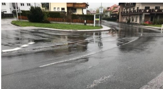
Figure 39: Standing water in the ruts (Source: Salzburg Research)
