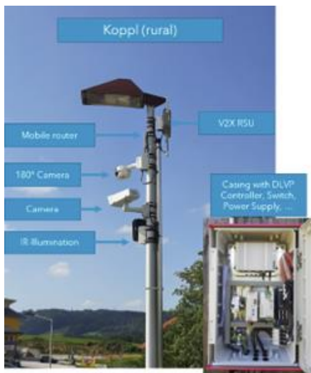
Figure 50: C-ITS installation on the pilot track for automated vehicles
