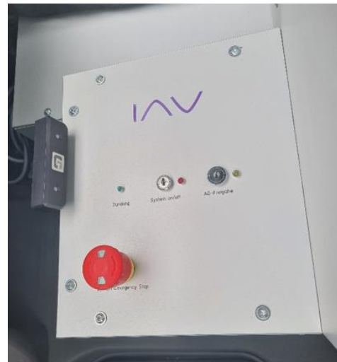
Figure 45: IAV operating and display panel for commissioning and decommissioning the measurement technology and the AD system ©DigiTrans GmbH
